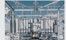
Transformer at the substation
