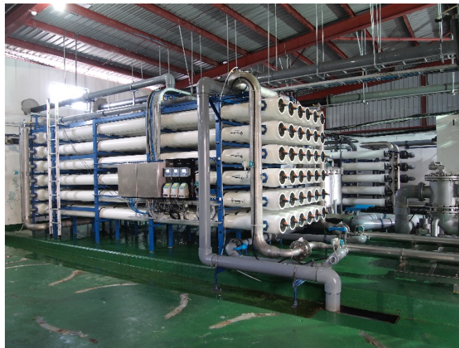
Hitachi Aqua-Tech's RO system (similar scale system for this project)
