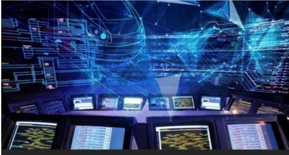
Signalling control centre
