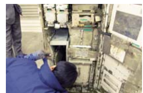
The tsunami caused major damage to 20 ATMs. Engineers tackled tasks such as repairing ATMs with case damage.
