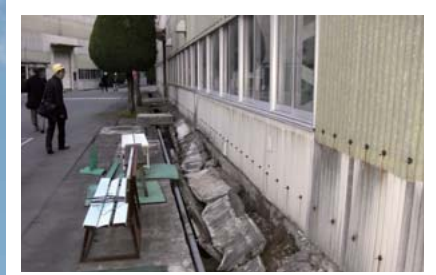
Hitachi Works after the disaster. Many Group factories were damaged.
