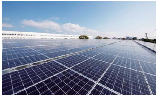
Photovoltaic system installed at Omika Works
