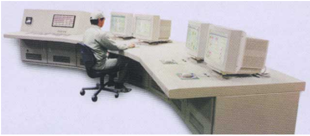
Fig. 1—New Supervisory and Control System for Radioactive Waste Treatment Equipment.
