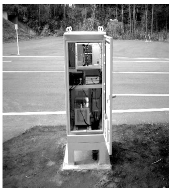
Fig. 9—Interior of the DSRC Wireless Base Station. Wireless base stations that conform to the DSRC wireless specifications (ARIB STD-T75), have been set up and communication experiments are being conducted.
