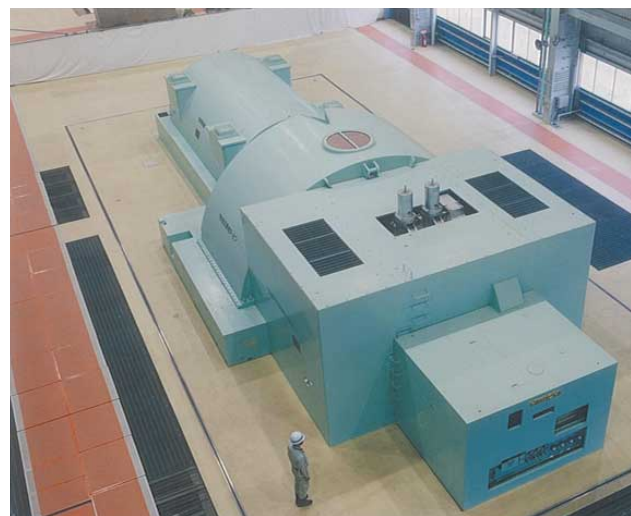
Fig. 2—Inside Turbine Room.
