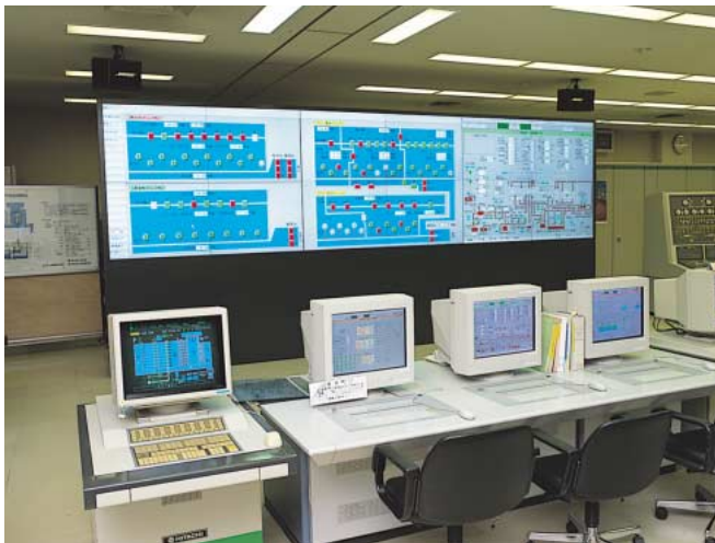
Large-display communication system delivered to sewage disposal plant of the Bureau of Sewerage, Tokyo Metropolitan Government
