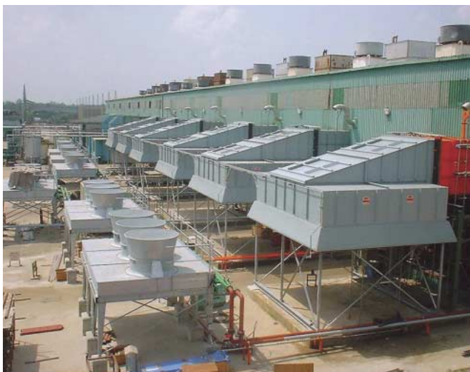
Outdoor View of the H-25 type gas turbines in Delta II Power Station
