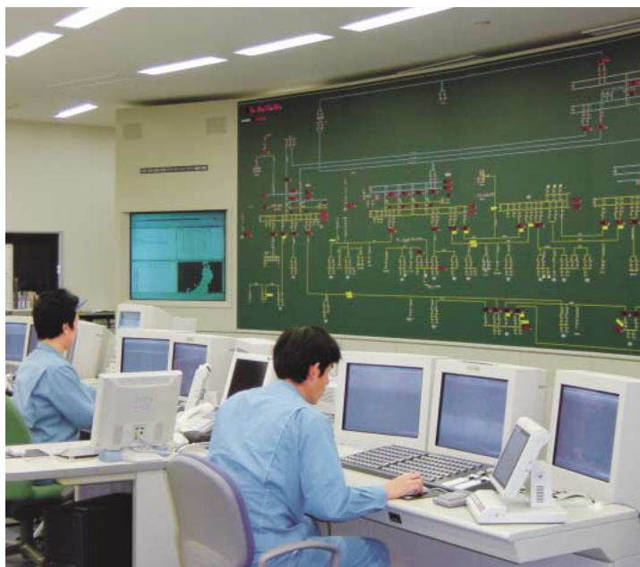
Power control and monitoring system delivered to Tohoku Electric Power Co., Inc.
