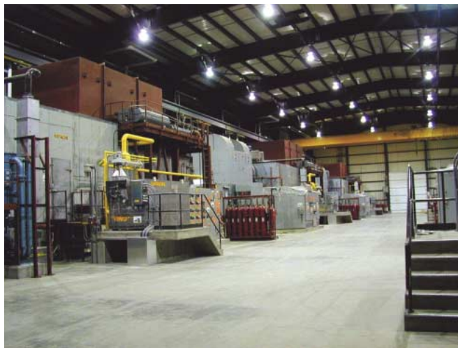
Indoor view of the H-25 gas-turbine units
