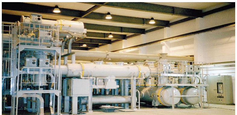
External view of 380-kV, 2,500-A/50-kA gas insulated switchgear at the JAMIA substation of the Saudi Electric Company in Saudi Arabia The switchgear is equipped with partial-discharge sensors so that preventive maintenance can be performed during operation by external diagnosis.
