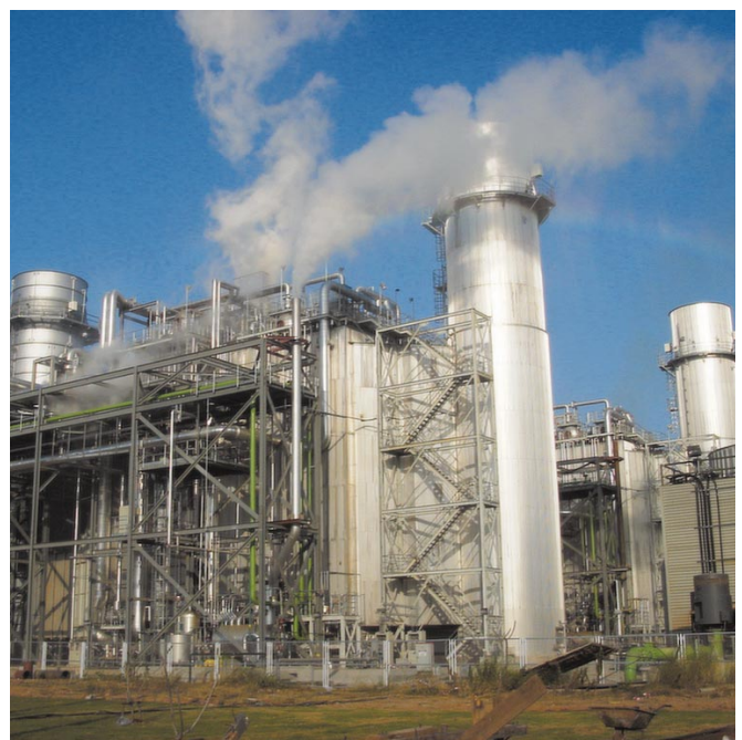
Overview of heat recovery steam generator for Ratchaburi Combined-cycle Power Plant Block-1
