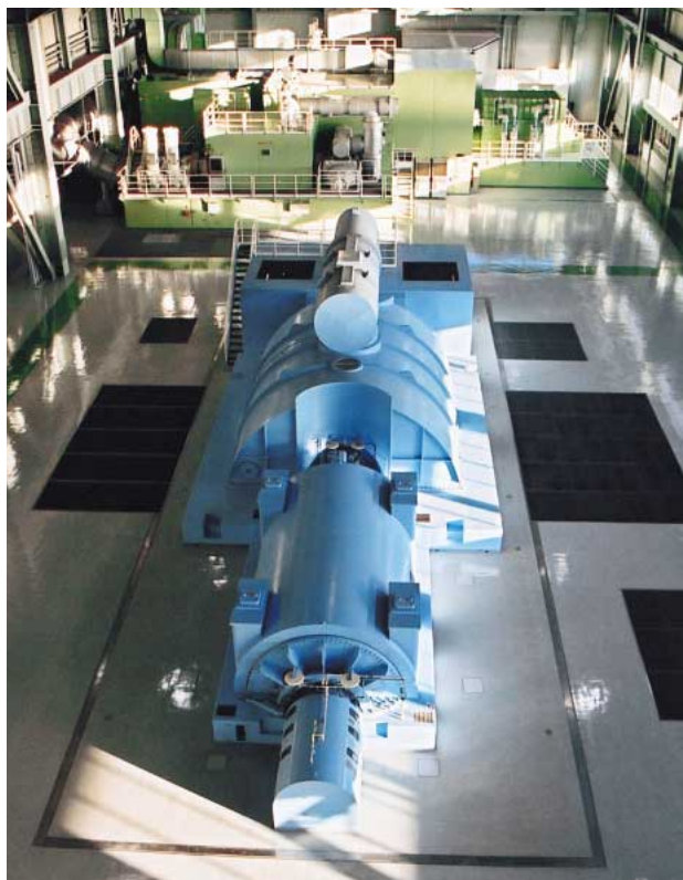
Fig. 3— Steam Turbine (Bottom) and Gas Turbine (Top) of the Power Station.
