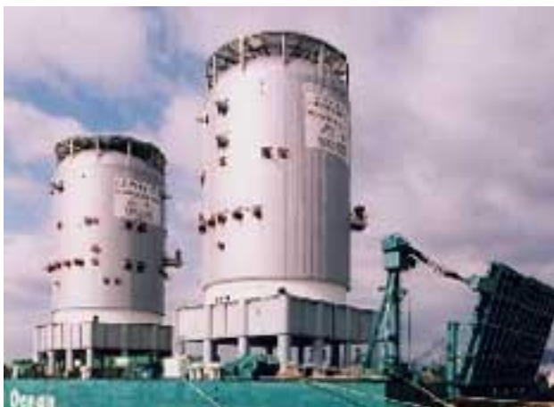
Fig. 2— Twin-Furnace Boiler (“W.B.”) of the Power Station.
