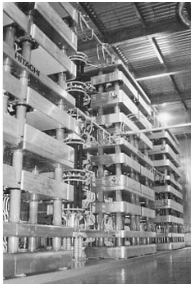
Fig. 6— A 700-MW Quadruple Multi-Valve Unit. The size per unit of electrical capacity was reduced to 60% of that of a conventional thyristor valve with 8-kV, 3,500-A direct-light-triggered thyristors.
