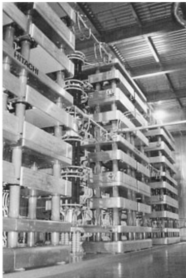
Fig. 6— A 700-MW Quadruple Multi-Valve Unit. The size per unit of electrical capacity was reduced to 60% of that of a conventional thyristor valve with 8-kV, 3,500-A direct-light-triggered thyristors.
