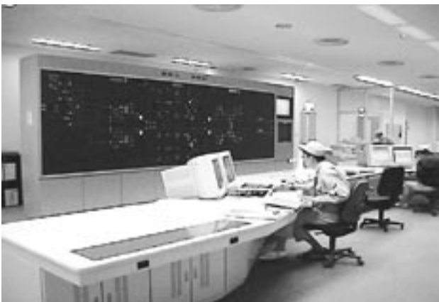
Fig. 9— Substation Control System of the Kihoku Converter Station.
