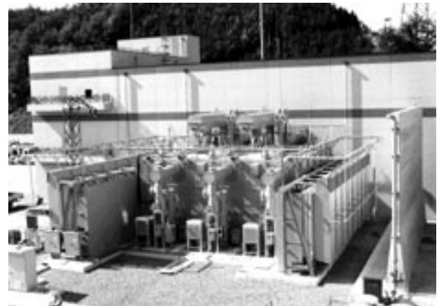
Fig. 7— 872-MVA Converter Transformer (Kihoku Converter Station).
