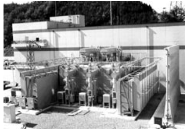
Fig. 7— 872-MVA Converter Transformer (Kihoku Converter Station).
