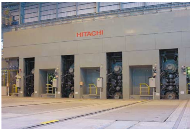
Tandem cold mill at Nisshin Steel
