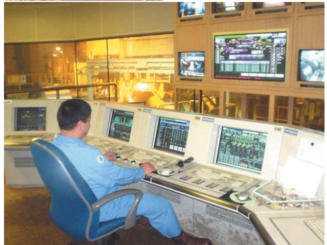
P2C equipment (above) and operation room showing one-person operation
