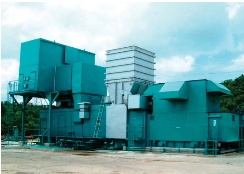
No. 8 type H-25 gas turbine power plant of Bahamas Electricity Corporation
