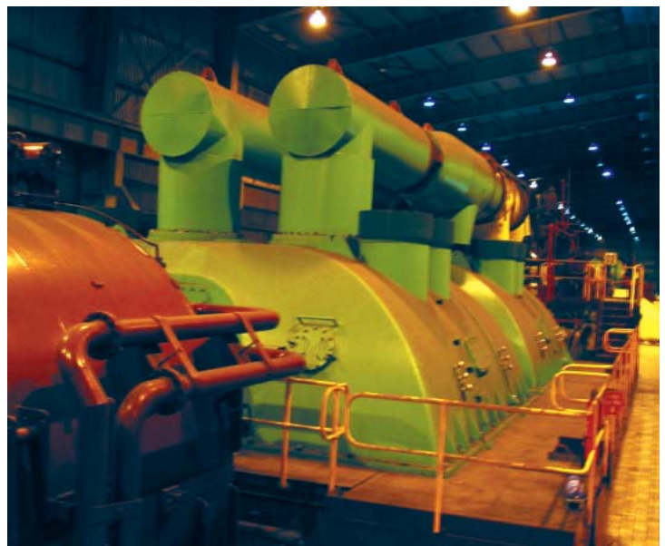
Indoor view of Macquarie Generation Liddell No. 2, Australia
