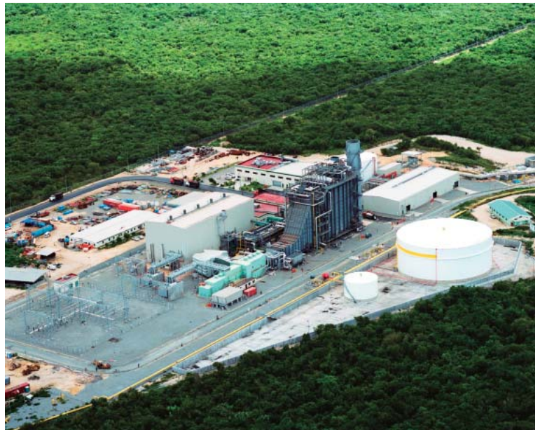
Overall view of AES Corporation's combined cycle plant
