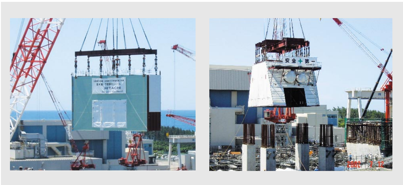
Fig. 1—Large Mobile Crawler Crane Lifts Lower Shell Block (left) and Upper Shell Block (right) onto Turbine Generator Base.
