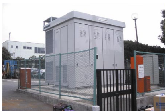
Fig. 6—External View of the 22-kV/6-kV Large-capacity Mini Substation. The new mini substation is already being delivered to The Tokyo Electric Power Co., Inc.
