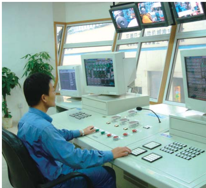
Central operation room
