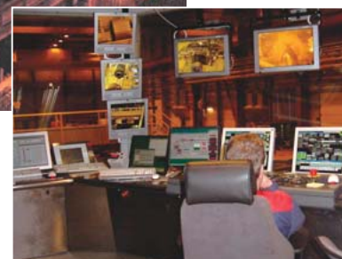
Finland's Outokumpu hot rolling mill electrical equipment (above) and operating room in action (below)
