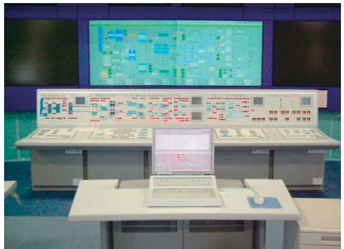
Central monitoring and control system at Niwakubo Water Treatment Plant, Osaka Waterworks Department
