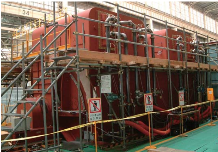
Performance tests of the generator at the test shop
