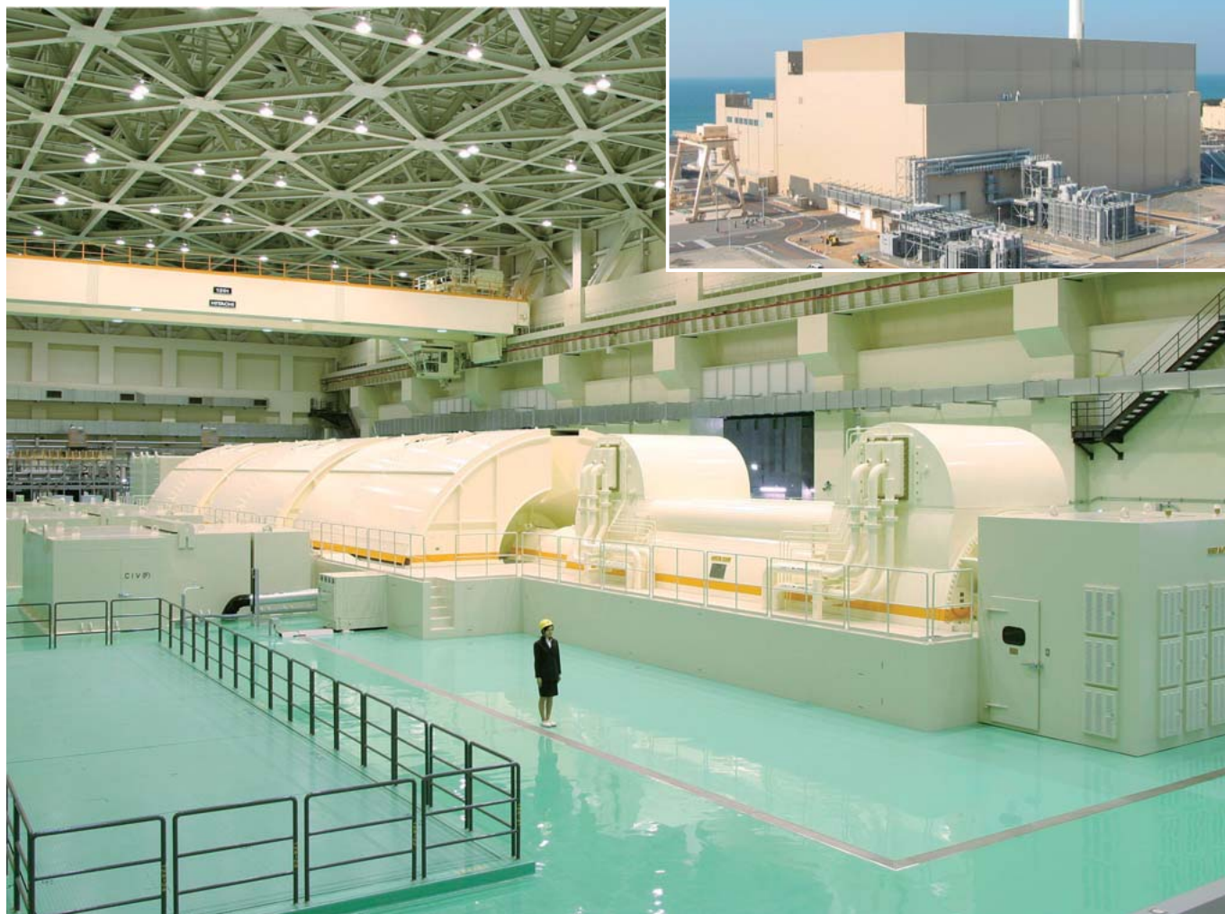
External views of the completed Unit No. 5 facility of Hamaoka Nuclear Power Plant (above right) and turbine generator (below)
