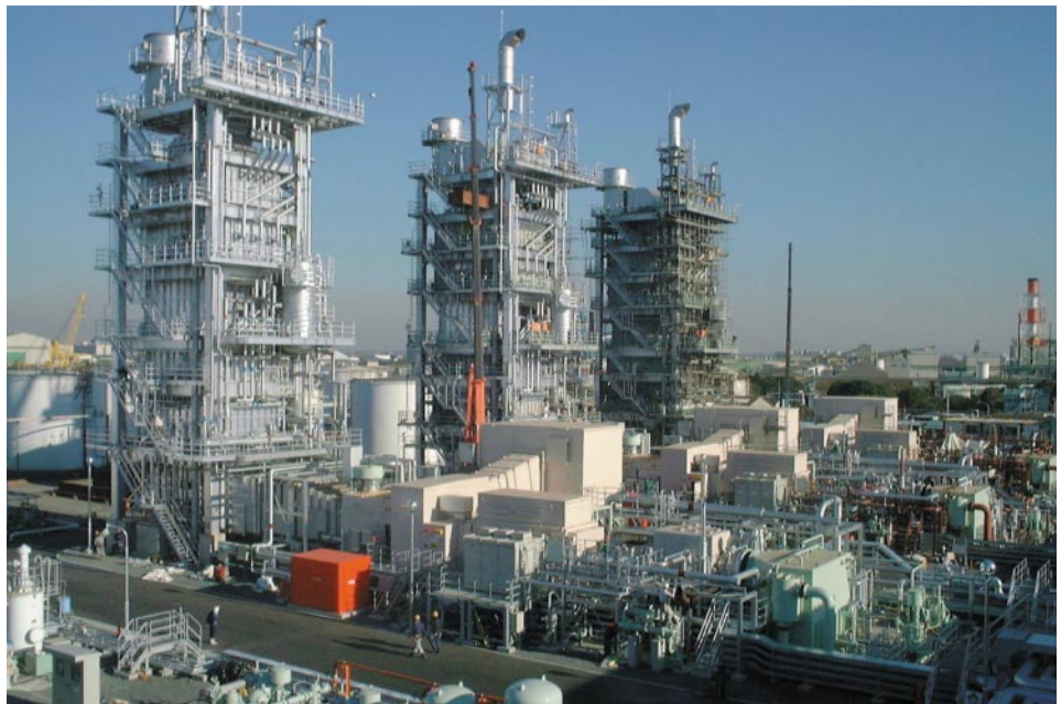
Fig. 1—External View of the Goi Power Plant of Goi Coast Energy, Ltd. Hitachi has completed three units of a single-shaft type combined-cycle power-generation plant on the premises of Chisso Petrochemical Corporation. Each plant consists of a gas turbine, generator, steam turbine, and heat recovery steam generator in a compact configuration.
