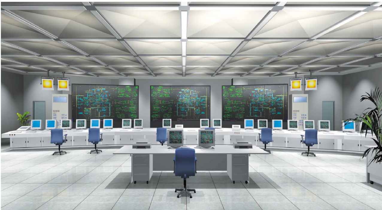
Fig. 1—Inside of Central Monitoring and Control Room Set up for New-generation Integrated Monitoring and Control System.
