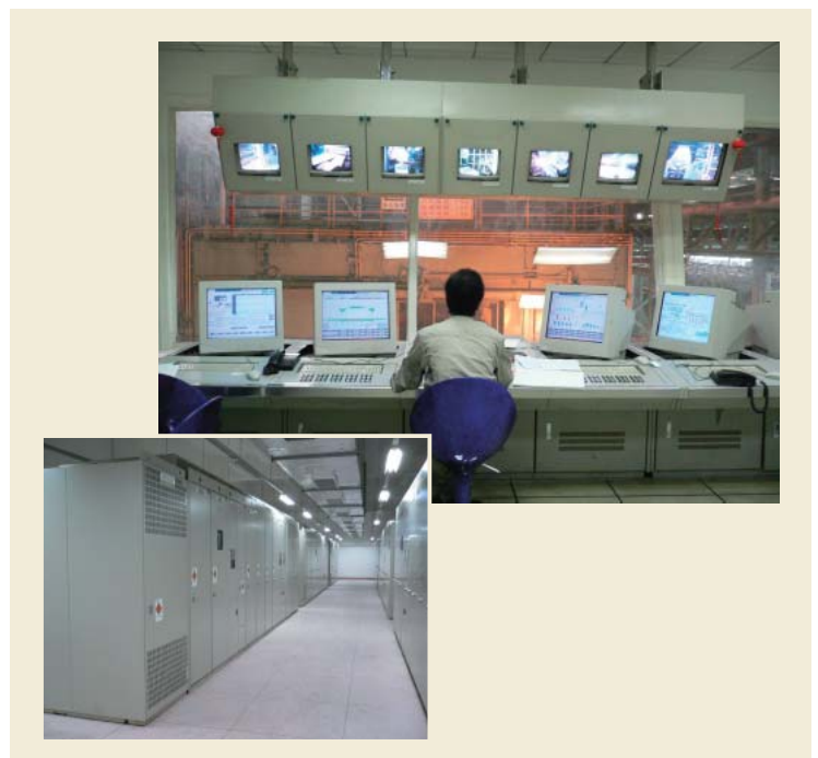
Central operation room (above) and high-voltage IGBT drive equipment (below)
