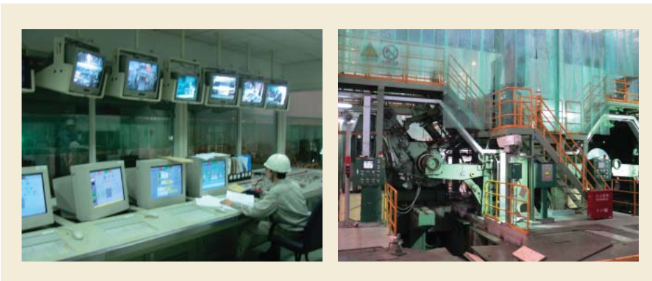
Operation control room (left) and delivery equipment (right)
