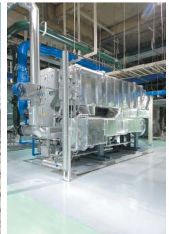
Steam absorption chiller
