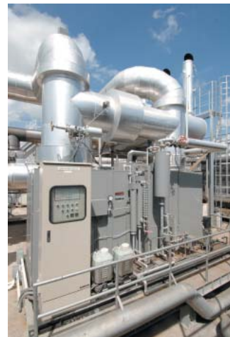
Exhaust heat steam boiler
