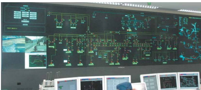
Projector-type integrated monitoring panel
