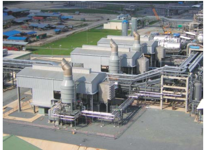
Full view of Betara Project gas-turbine generator sets
