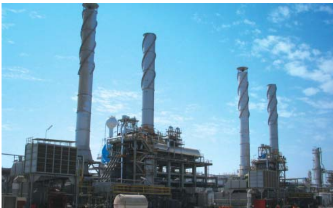
Overview of H-25 gas-turbine sets delivered to the Sohar Oil Refinery of the Sultanate of Oman
