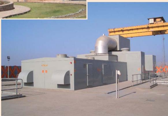
Full view of Cairo North Power Station (top) and steam-turbine generator (bottom)
