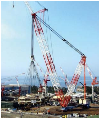
Construction of ABWR (Unit 2 of the Shika Nuclear Power Station of Hokuriku Electric Power Company)
