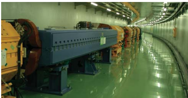
50-GeV synchrotron electromagnets installed inside tunnel
