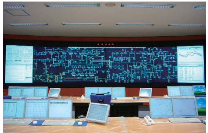
Video projection system screen and operator consoles in dispatching room
