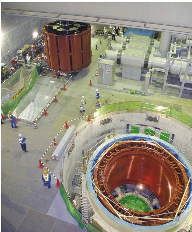
Fig. 3—Generator-motor Stator and Rotor.
