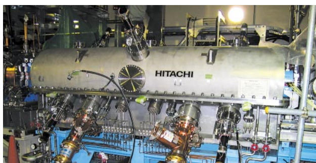
Fig. 2—RFQ Installed at the Linac Wing.
