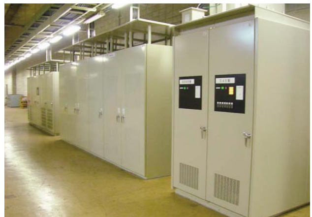
Fig. 1—Photo of the Regenerative Power Absorbing Equipment Using Batteries in Operation (Kobe Subway, Seishin-yamate Line, Itayado Substation).
