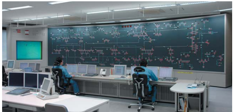
Aomori Regional Load Dispatching Center
