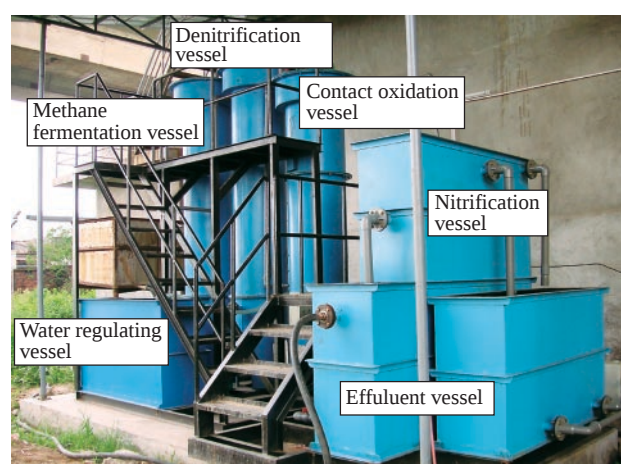
Fig. 5—Pilot Plant for High-concentration-ammonium Effluent Treatment.
