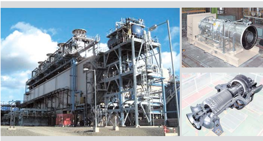
Fig. 1—H-25 Gas Turbine and General Overview of Sakhalin II Project in Russia.
