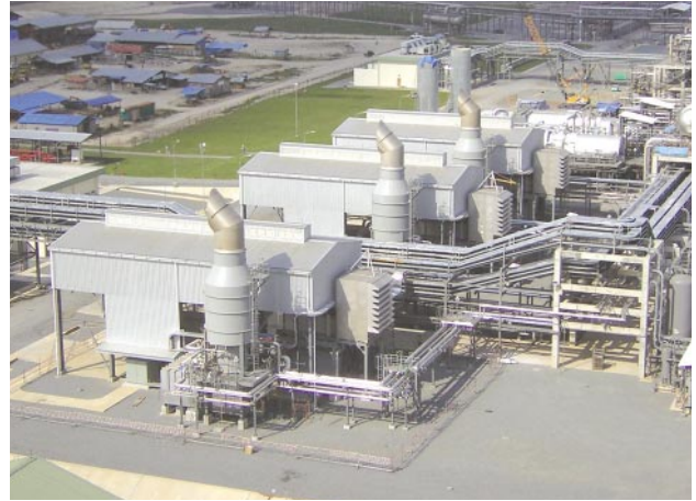
Fig. 7—Overview of Betara H-25 Plant. Hitachi delivered three H-25 gas turbine generator sets to Betara plant in Indonesia.
