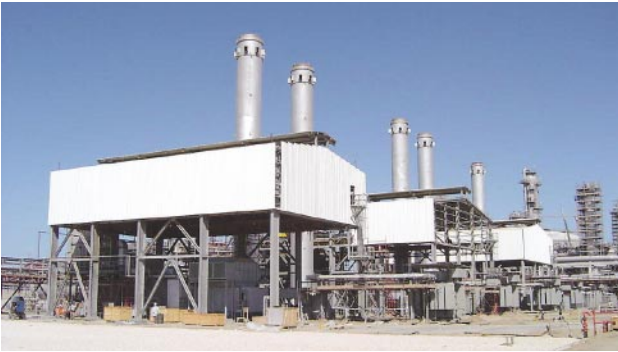
Fig. 6—Overview of Damietta H-25 Plant in Egypt. Hitachi delivered five H-25 gas turbine generator sets to Damietta LNG plant through Kellogg, an engineering company.
