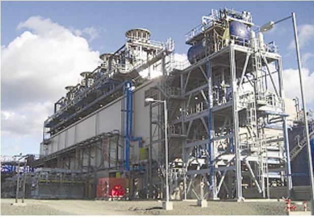
Fig. 5—H-25 Gas Turbines in Sakhalin II Project in Russia. Hitachi delivered four H-25 gas turbine generation equipment units to the Sakhalin Energy Investment Co., Ltd., for use in a land-side plant that processes gas and oil extracted from the seabed off the eastern shore of Sakhalin Island in Russia.
