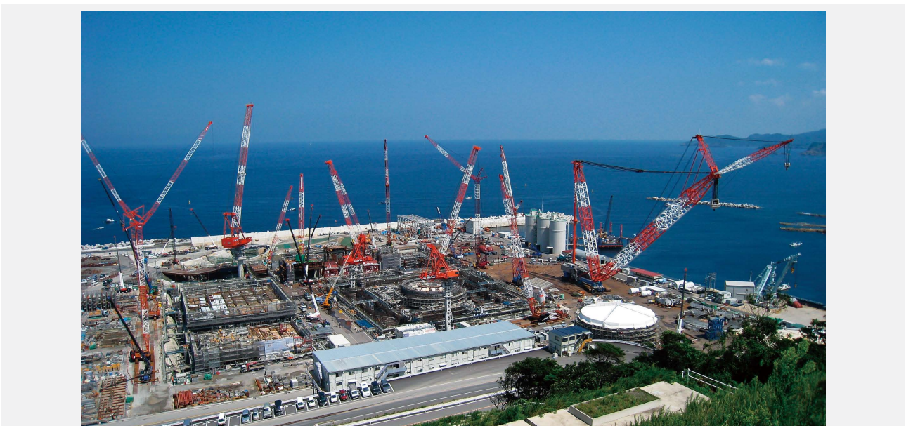
Fig. 1— Construction of Unit No. 3 at the Shimane Nuclear Power Station of The Chugoku Electric Power Co., Inc. The plant is being constructed using the latest construction methods including the large crawler crane at the right of the photograph. Equipment installation is now in progress with building and equipment construction proceeding in parallel.
