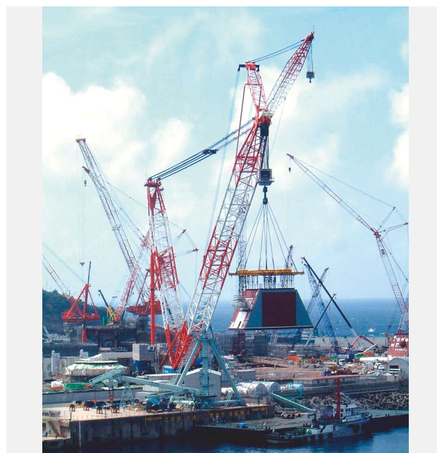
Fig. 4—Direct Unloading by Large Crawler Crane. The large crawler crane unloading (lifting) the upper body module of the condenser is shown.
