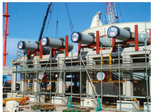
Fig. 2—RCCV Interior Module (Upper Dry Well). The on-site assembly of an RCCV (reinforced concrete containment vessel) interior module is shown. The total mass is approximately 650 t.
