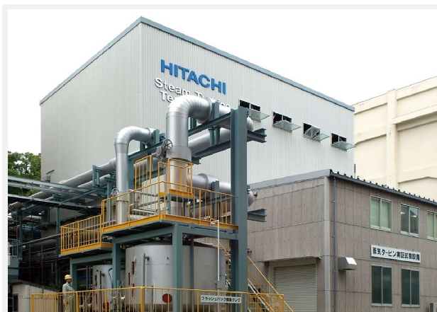
Fig. 6—Steam Turbine Test Facility. Trials can be performed using a model turbine that simulates an actual turbine.
