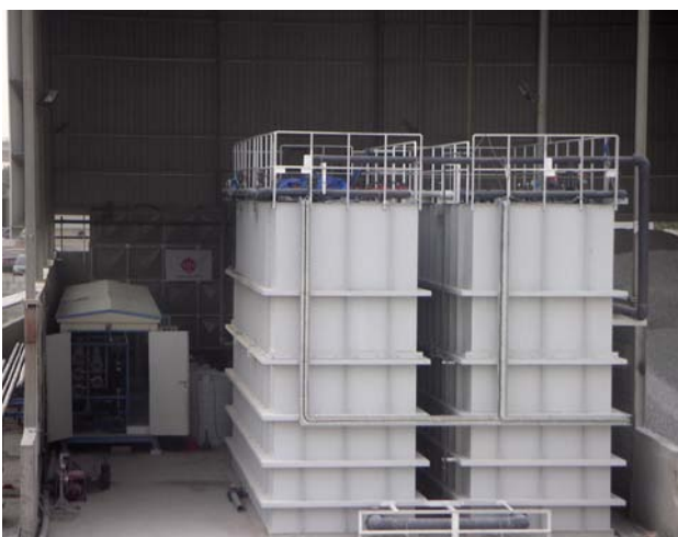
Fig.7—First Stage Plant of Water Recycling Project.
