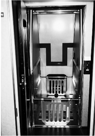
Fig. 7— Lifting Equipment for Wheelchair. The picture shows the lifting equipment for raising people using wheelchairs to the second floor. It can also be used for vending carts.
