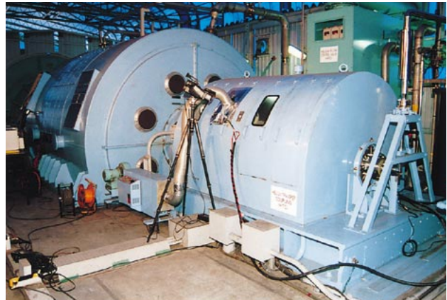
Fig. 2—70-MW Class Superconducting Generator in the Super-GM Testing Center.
