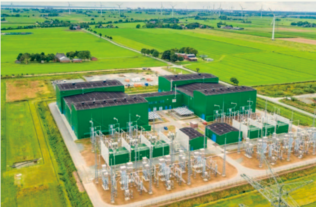
NordLink, a \pm 525 -kV/1,400-MW and about 600-km HVDC link that connects Norway and Germany
