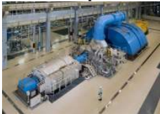
Turbines and generators
