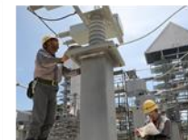
Maintenance and service
