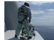
Maintenance and service
