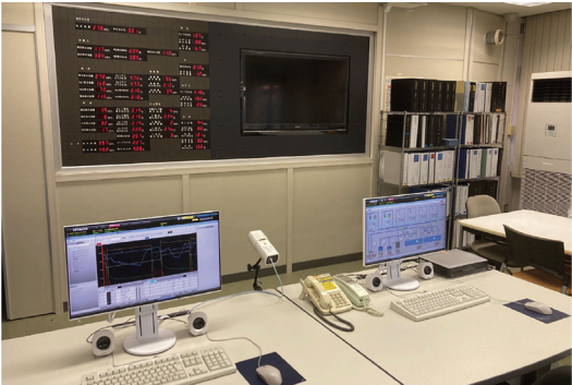
[01] Water Supply Facilities Central Monitoring and Control Equipment at Higashine City Hall, Yamagata Prefecture
