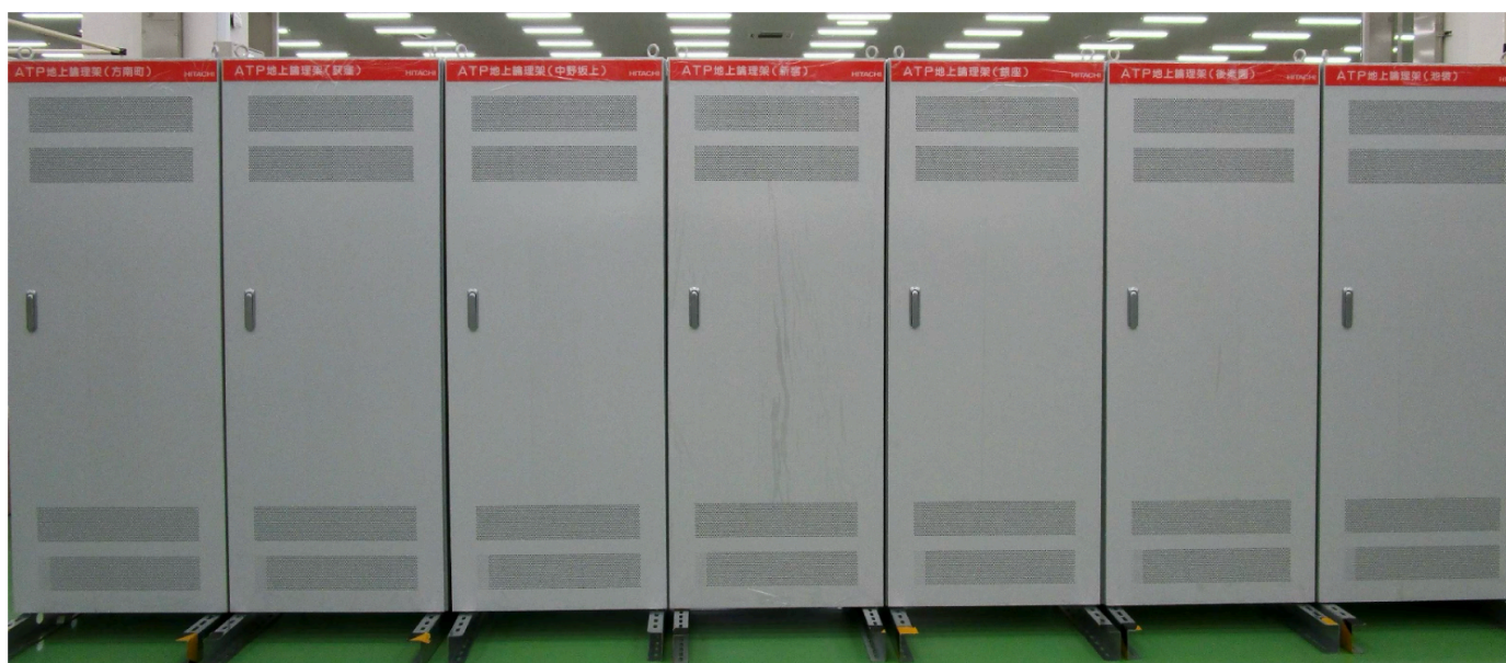
[2] Wayside Automatic Train Protection systems for the Marunouchi Line
