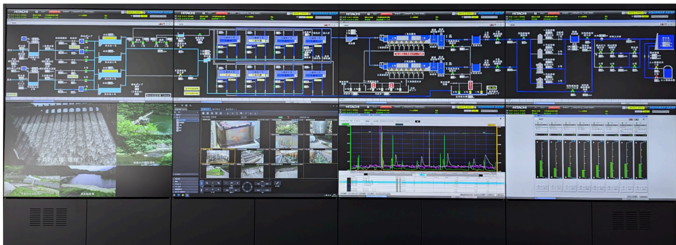
[3] Use of Wide-screen Display for System-wide Monitoring
