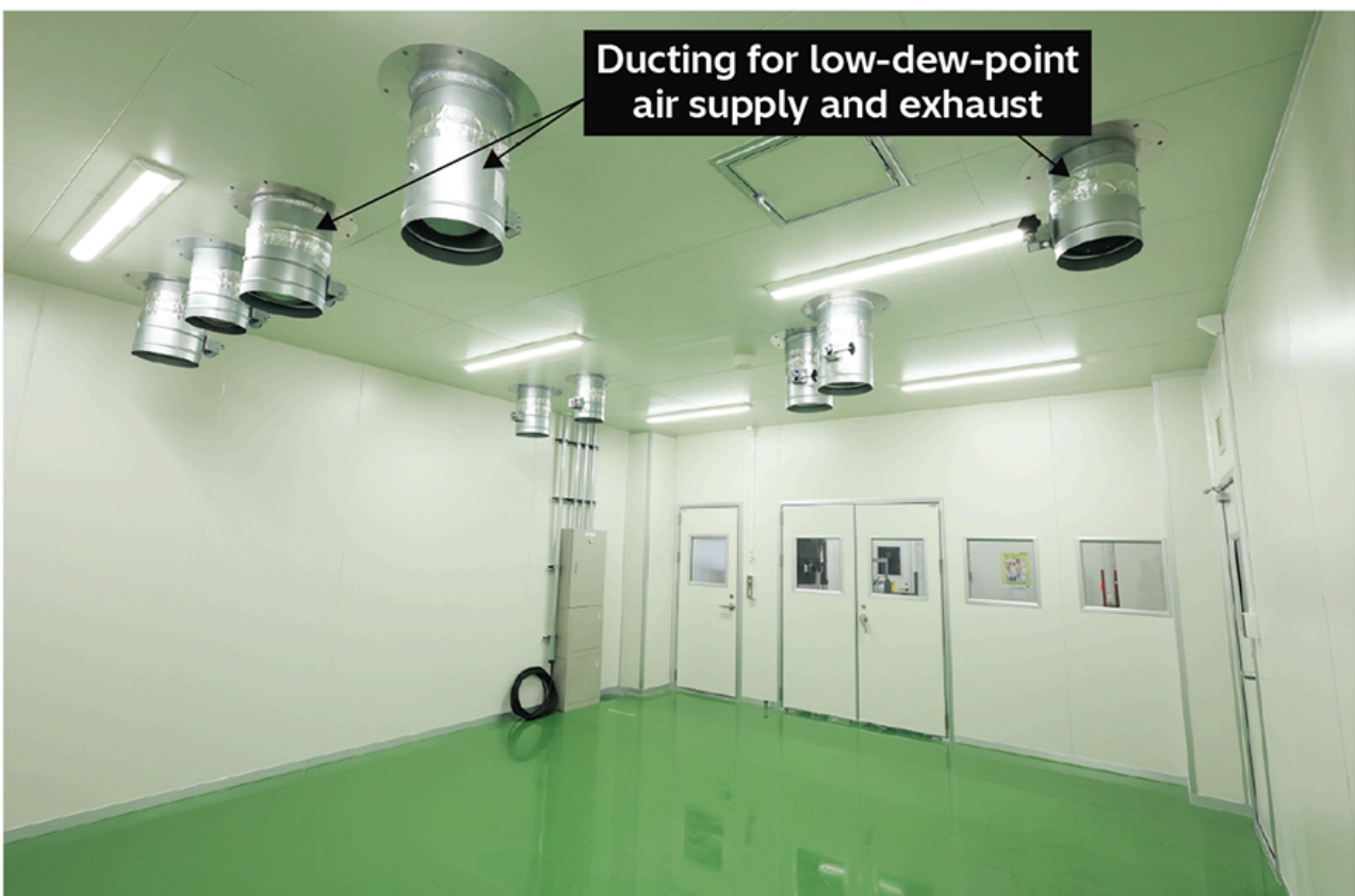
[7] Interior of Test Chamber with Variable Dew-point Temperature
