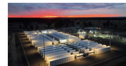
Ulinda Park BESS, Queensland, Australia
