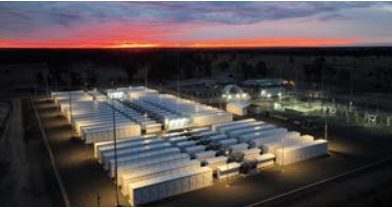
Ulinda Park BESS, Queensland, Australia
