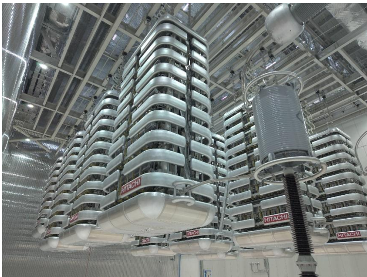
Valves hall at the converter station in Mumbai
