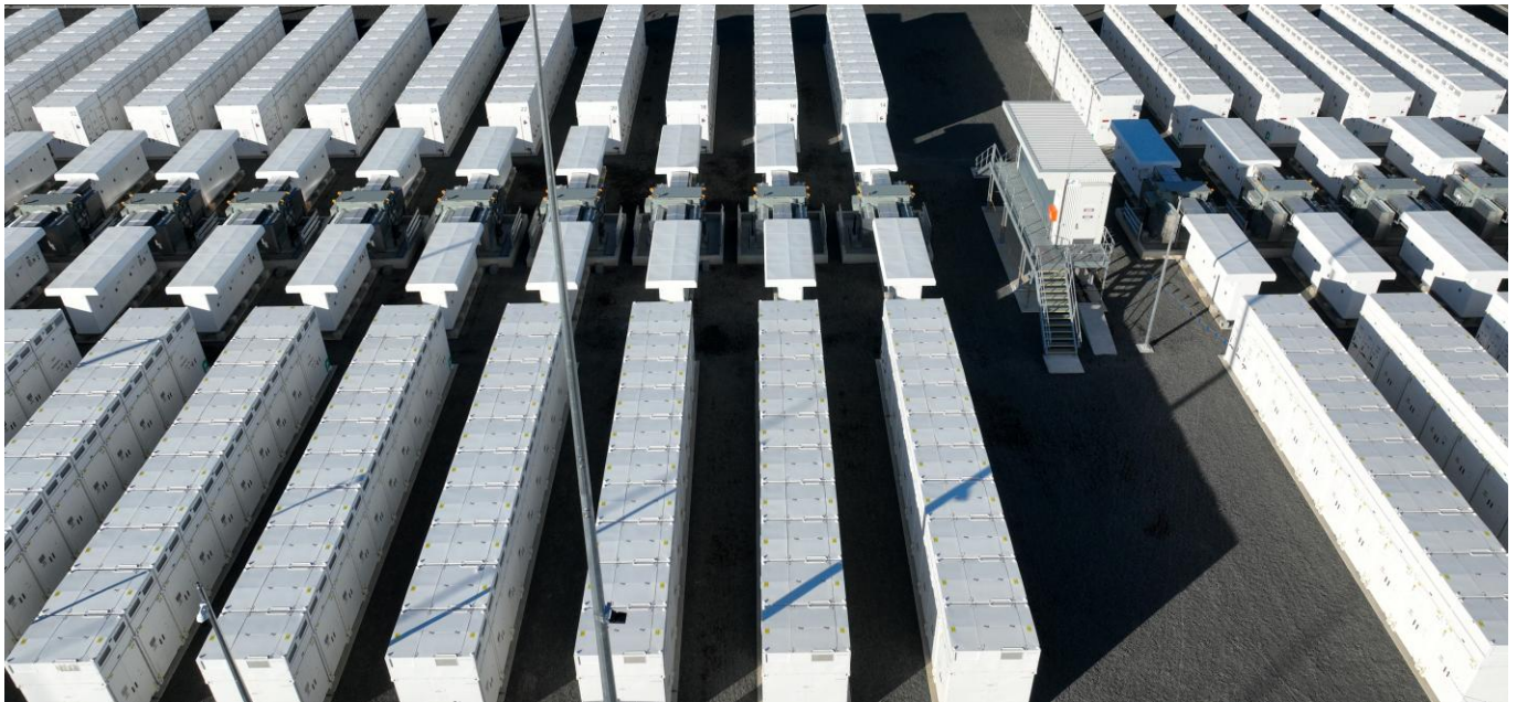
Ulinda Park BESS in Queensland, Australia
