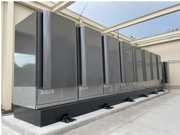
Fuel cell system under demonstration at Hitachi's Omika Works
