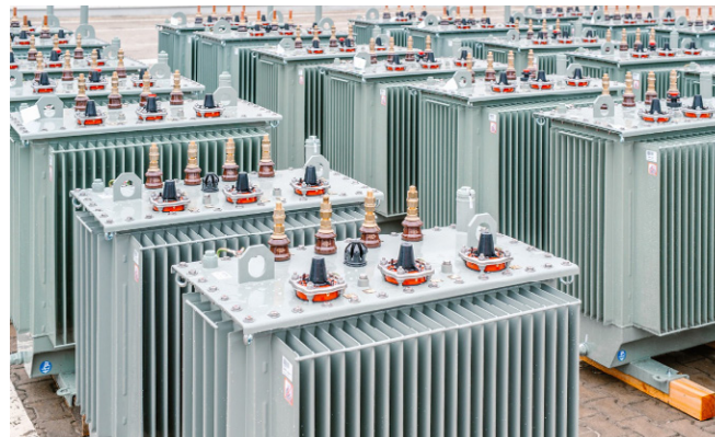
Recycled mineral oil-filled transformer
