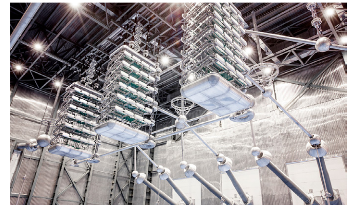
High-voltage direct current (HVDC) transmission system
