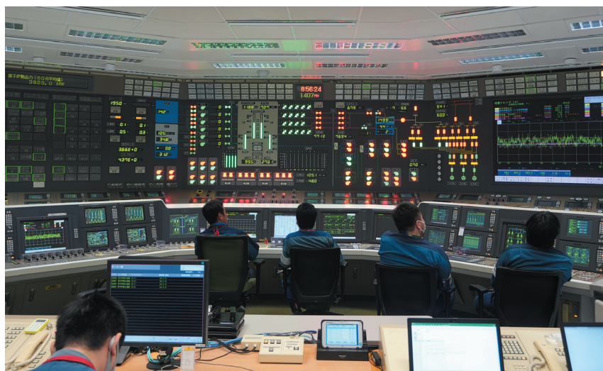
Main Control Room. The main control room is where the status of the nuclear reactors, turbines and generators, etc. are monitored, and their operation is controlled (photo courtesy of Tokyo Electric Power Holdings, Incorporated)
