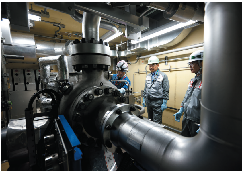
The high-pressure alternate cooling system (HPAC). The system is able to inject water into the reactor without using electricity during an emergency.
