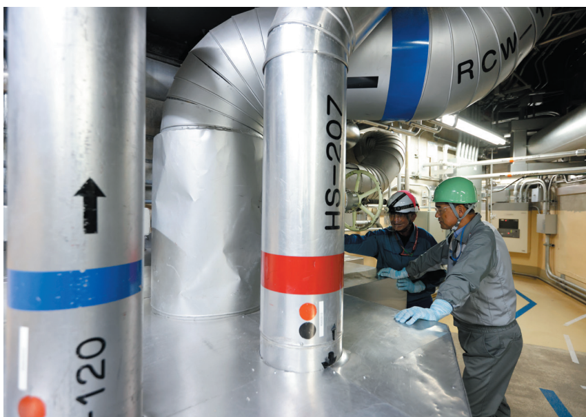
Handles in various locations are coated with phosphorescent paint to make identification easier in the dark.
