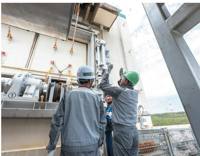
Blowout panels and large winch of the forced-opening equipment
