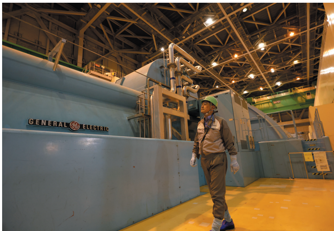
Unit 6 has an output of 1,356 megawatts (the same output as Unit 7), and the turbine building generates large amount of power equal to that consumed by 450,000 average households.
